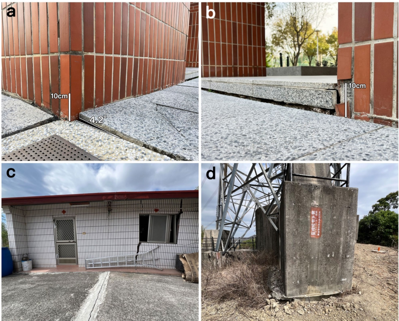
Fig. 1. The damaged buildings and infrastructures due to land surface deformation. (a,b) Uniform surface deformation leads to buildings separating from surrounding ground facilities, causing damage that is very common in SW Taiwan. However, (c,d) in regions with high deformation rates, severe land surface deformation can significantly damage the structures of buildings and infrastructure (e.g., transmission towers), raising safety concerns.
